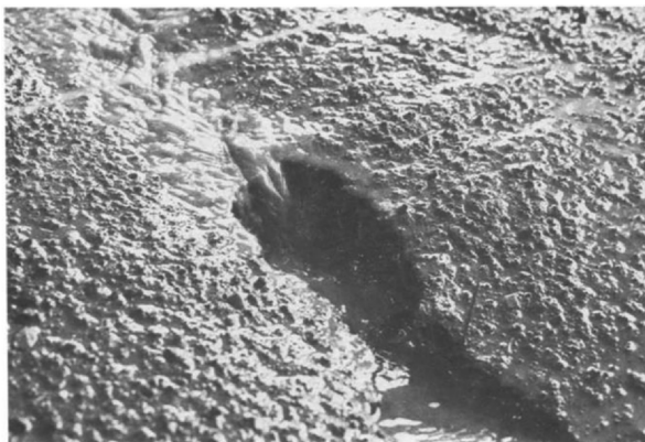
Fig. 3. Typical scoured knickpoint (Merz and Bryan, 1993).
