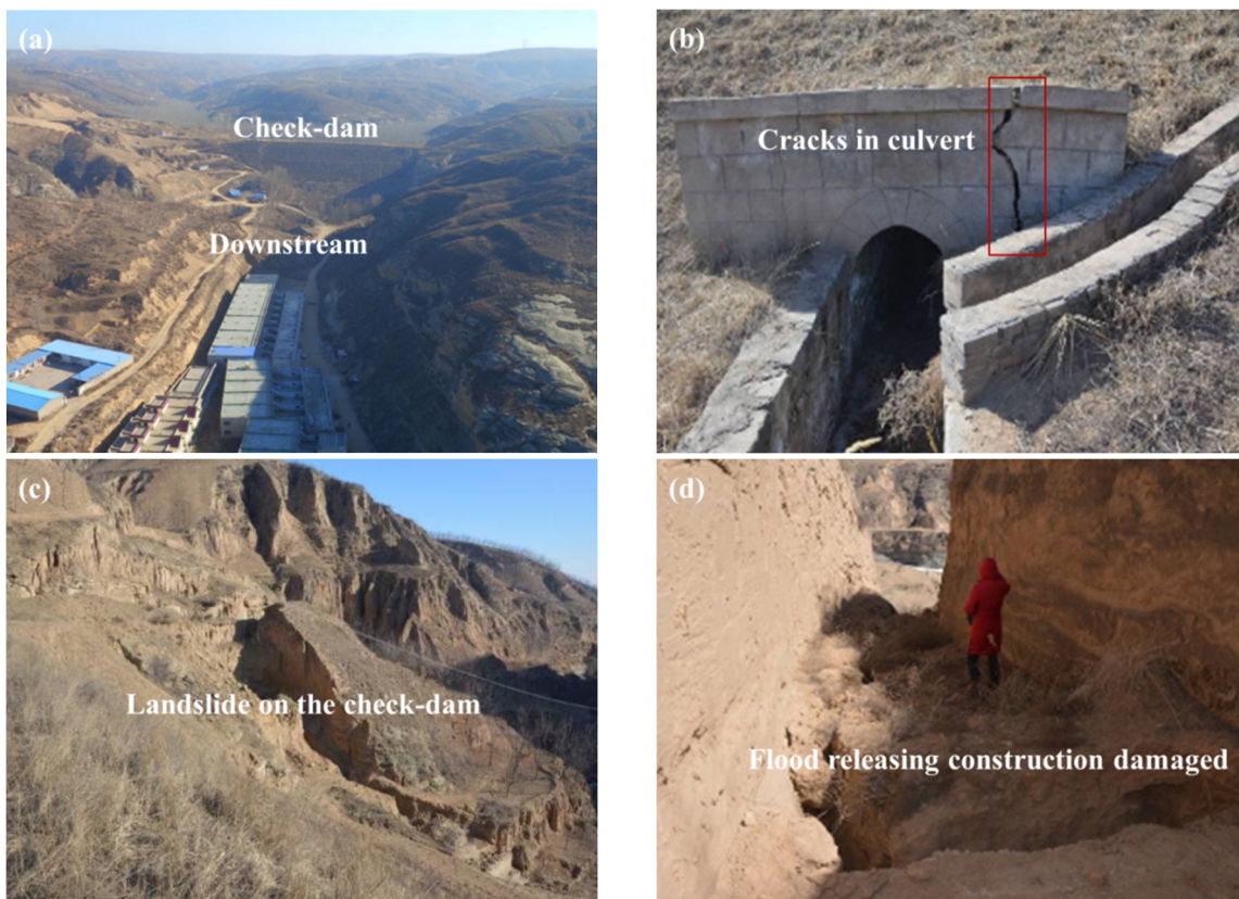
Fig. 4 The different dangerous situation of check dams on the Loess Plateau in China. (a) There were some important facilities located 300 m at the downstream of the check-dam. (b) There was a crack in the culvert of the check-dam. (c) A landslide occurred at the dam body of the check-dam. (d) Flood releasing construction of the check-dam damaged.
